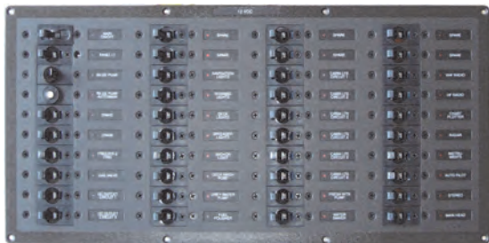
AC & DC Electrical Panels
